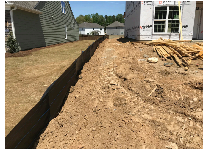
Physical barriers such as silt fencing are an effective erosion control measure in land development.
